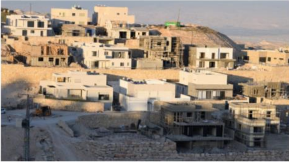
A construction site of a new residential neighborhood at the mixed religious-secular Jewish settlement in the West Bank Kfar Adumim, March 9, 2023. (Gili Yaari /Flash90)
